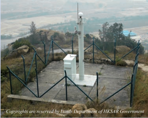
Siu Lang Shui Satellite Positioning Reference Station
