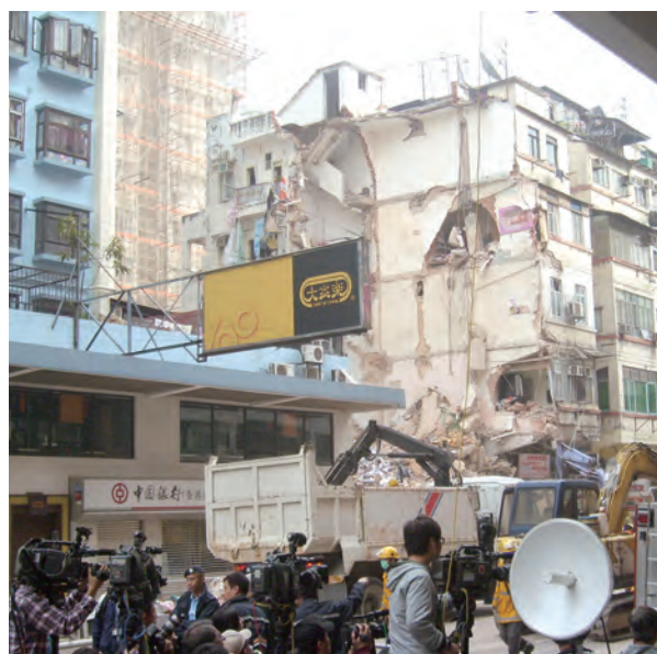
Scene after the tragedy of collapse at 45J Ma Tau Wai Road on 29 January 2010.
