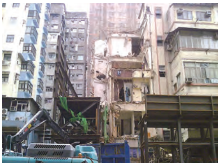
Strengthening and temporary works were installed to 45J & 45H Ma Tau Wai Road before the Chinese New Year.
