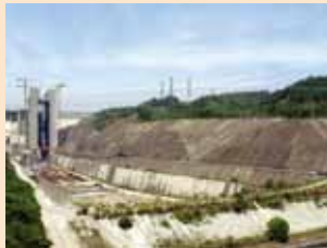
The ship lift under construction with the cover dam at the front.
