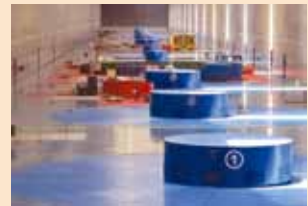
The Power-plants inside the Power Station
