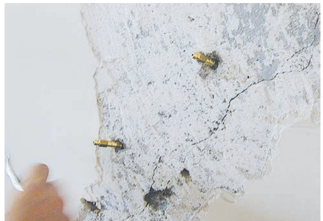
Injection packers drilled into the concrete on both sides of the identified crack
