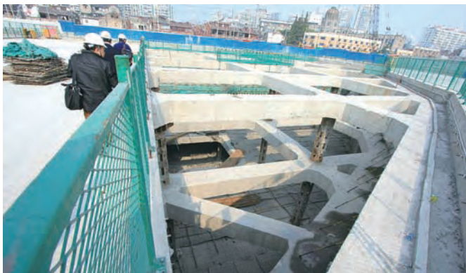
Preparation for demolition by explosion of temporary concrete support for deep excavation was in progress.
