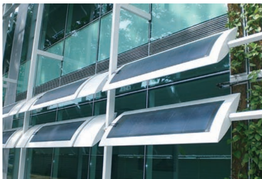
Figure 2: 2nd Generation PV Modules installed on Sunshades
