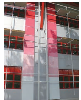
Figure 17: Ventilation Ducts connected to the Solar Chimneys ►
