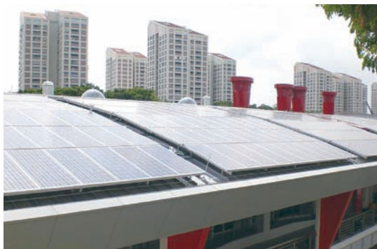
Figure 1: 1st Generation PV Modules installed on Roof
