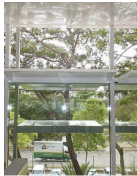
Figure 12: Sunshade, installed below the light shelf to reduce glare into the building
