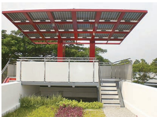
Figure 3: 3rd Generation PV Modules installed on Canopy
