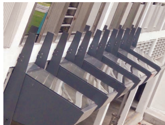
Figure 6: Mirror Duct System installed on the Façade of the building
