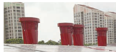
Figure 16: Solar Chimneys installed on the Roof of the Building ▲
